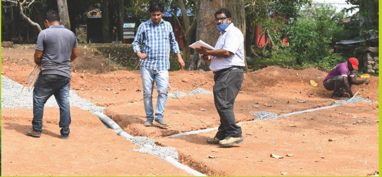
Late. Murari, Asst. Engineer CPWD, Shri. Kamal and workers during the Up Gradation works of 3rd And 7th Green
